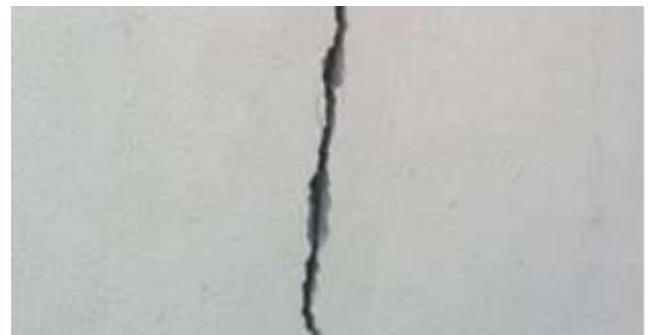
Fig 1. Crack on the wall Width: Above 5mm Type: Wide Crack
