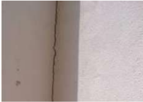
Fig. 2. Crack at the corner Width: Above 2mm Type: Wide Crack Probable Causes: Temperature Variation or Shrinkage
