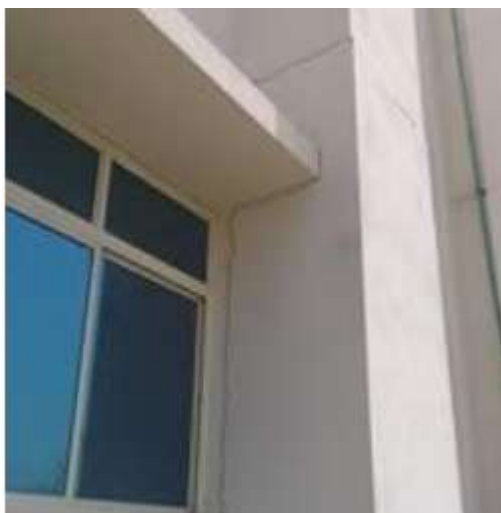
Fig. 4. Crack above window Width: Between 1 to 2mm
