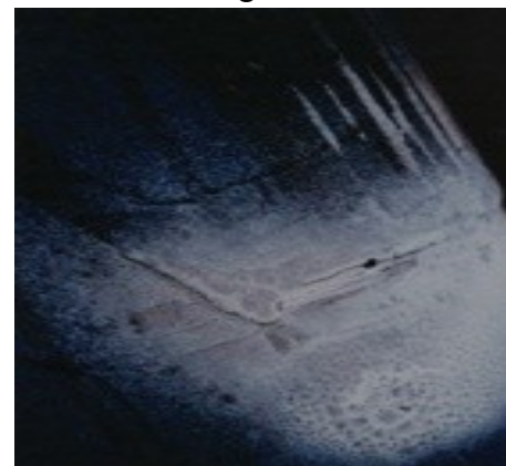
Crack in fillet welds
